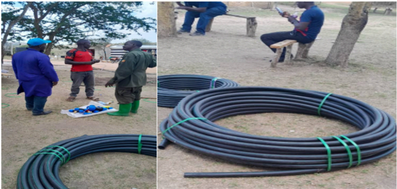
Figure 46-47: Water installation to facilitate a tourism product at Lake Mbuoro National Park
